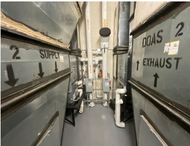
27 - HEAT PUMP ROOM
