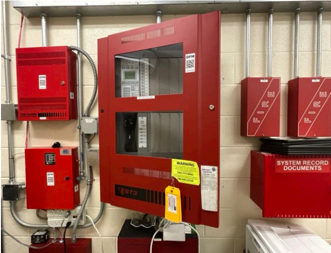
25 - FIRE ALARM PANEL
